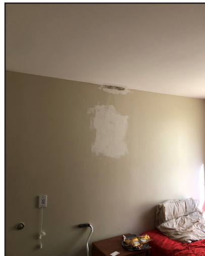
Figure 6 – At BFNC: water damage from a ceiling leak.
