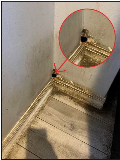
Figure 3 – At Federation: evidence of vermin in unit.
