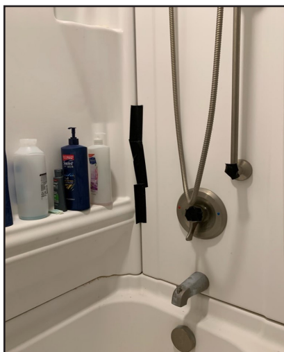
Figure 5 – At DePaul: leak in shower that went unaddressed and had to be duct-taped by the resident as a fix.
