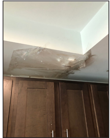
Figure 2 – At Community Access: active leak in a kitchen, taped over with plastic as a temporary fix.
